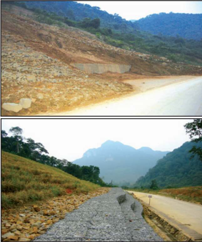
Photo 27: Da Deo Pass, Quang Binh: Upper: Vegetation cover is destroyed, revealing ugly and continuous failures of cut slopes; lower: Vetiver rows on top of the slope very slowly squeeze down, considerably reducing the failed mass.
