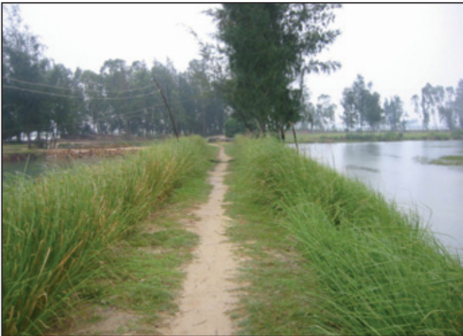
Photo 11: Vetiver grass planted on river dike along Tra Bong River (upper) and lining the sides of an anti-salinity estuary dike along the same river (lower).
