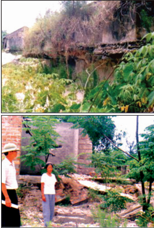
Photo 2: Sand flow in Le Thuy (Quang Binh) in 1999: the foundation of a pumping station (upper); this woman's three-room brick house is collapsing because sand has been blown from foundation (lower).
