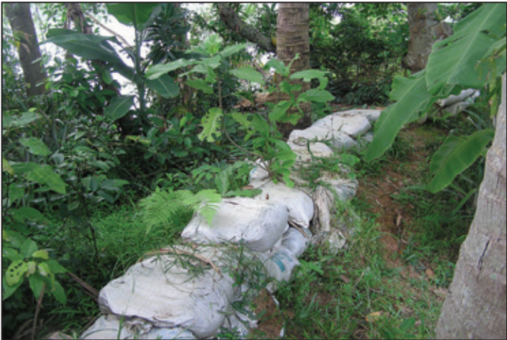
Photo 12: Upper: severely eroded bank of the Tra Khuc River, at Binh Thoi Commune; lower: primitive sand bag protection.
