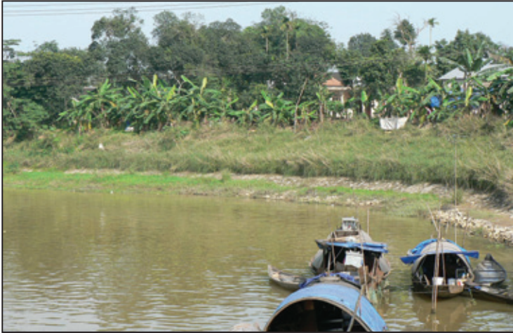
Photo 10: Upper: Vetiver and rock riprap and concrete frame protect an embankment; lower: a bend on Perfume River bank in Hue - protected with vetiver.
